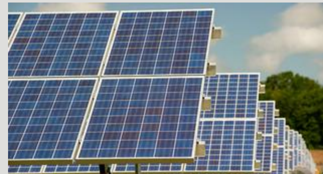
Solarpark Starwood, Canada
