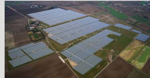
Solar power plant: Strasskirchen, Germany
