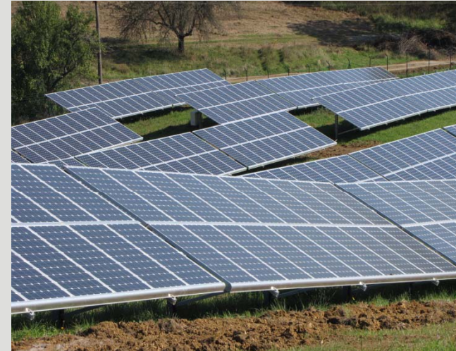
C&I system (greenfield): Uzovská Panica
